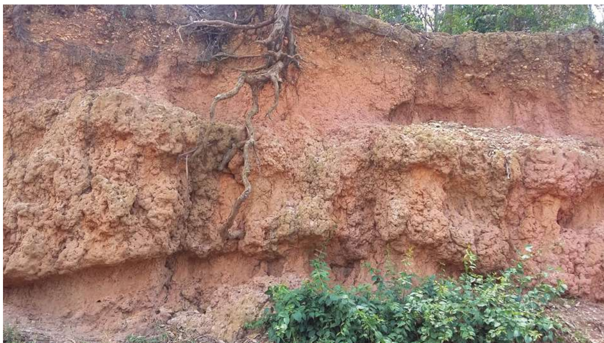
Plate 1: Eroded road side in Kihiihi Sub-county
