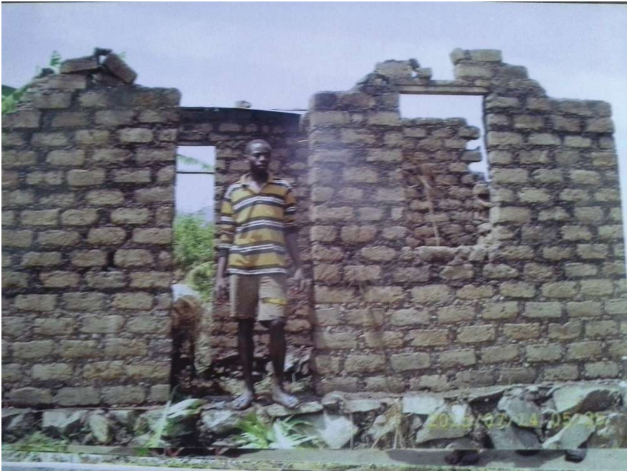
Plate 5: House that was destroyed by strong winds in Mpungu Sub-county
